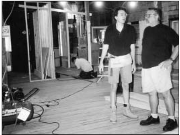
RCS Jefe, Hank Auderer, directs contractors at the new lab at 5103 McCullough. Hank has been actively participating in the demolition and construction.
